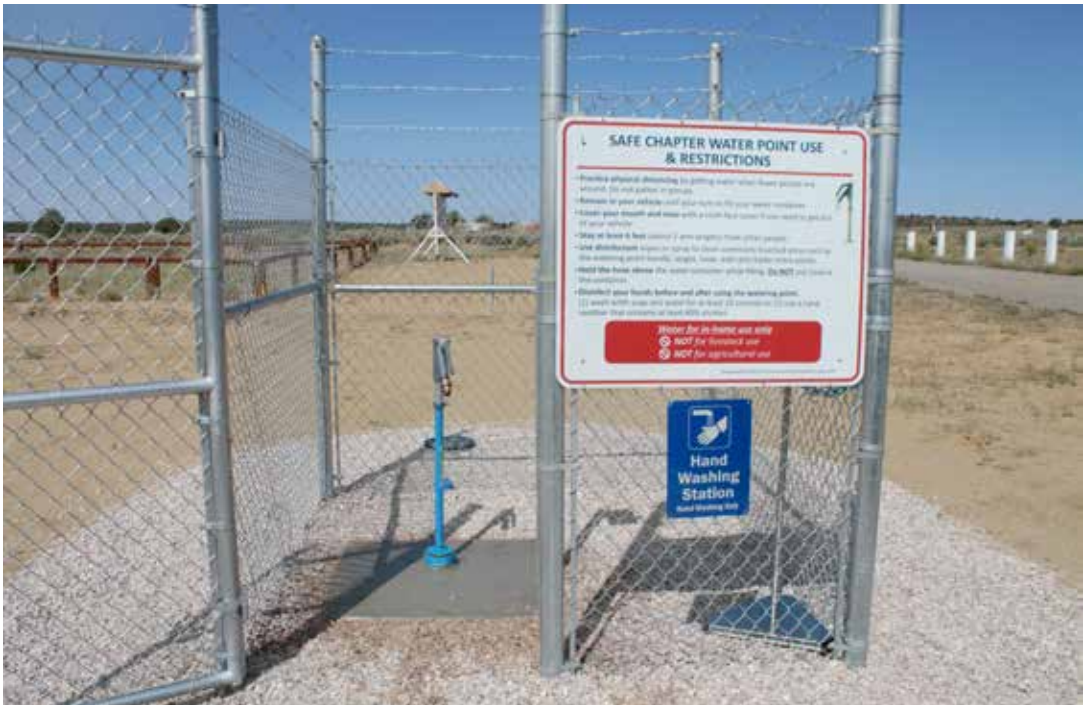
A newly installed transitional water point on the Navajo Nation, one of 59 constructed during the COVID-19 pandemic. Photograph by Nikki Tulley.
